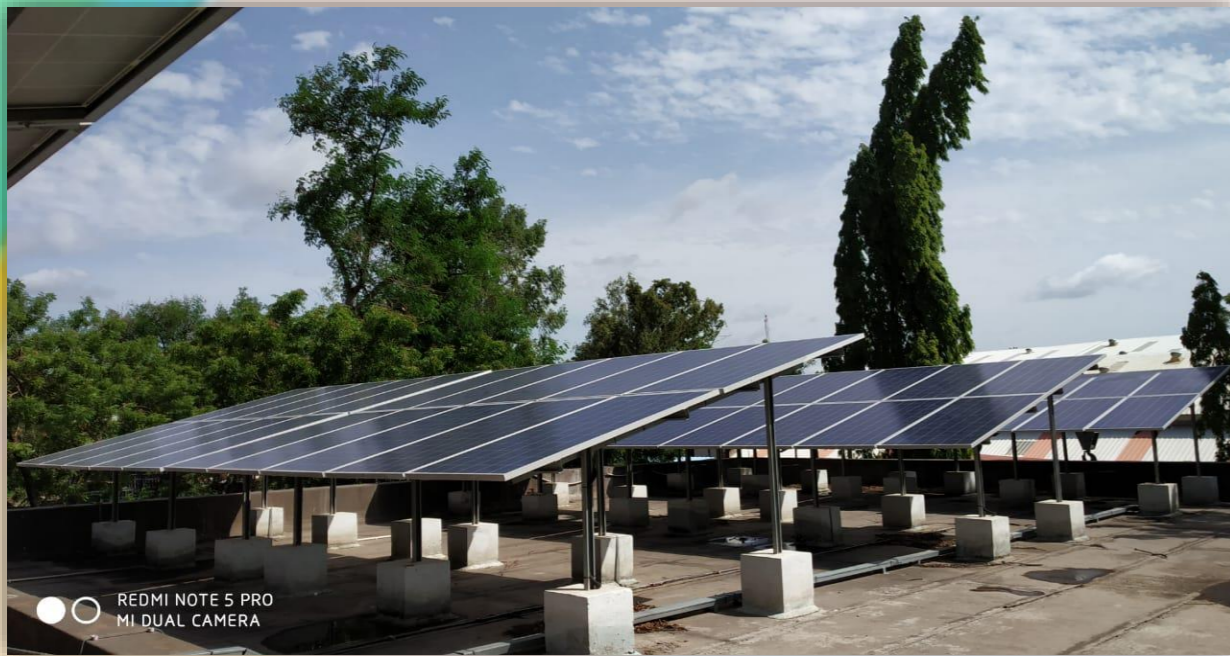
Rooftop Solar Plant- A substation
