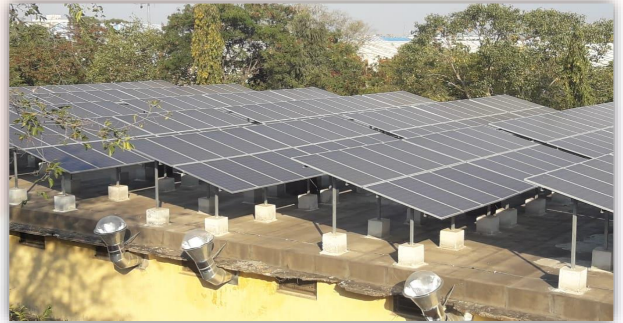
Rooftop Solar Plant- CMT Lab
